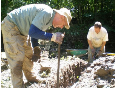
Chauncy Young and Larry Fisher digging one of several trenches for the foundation.
